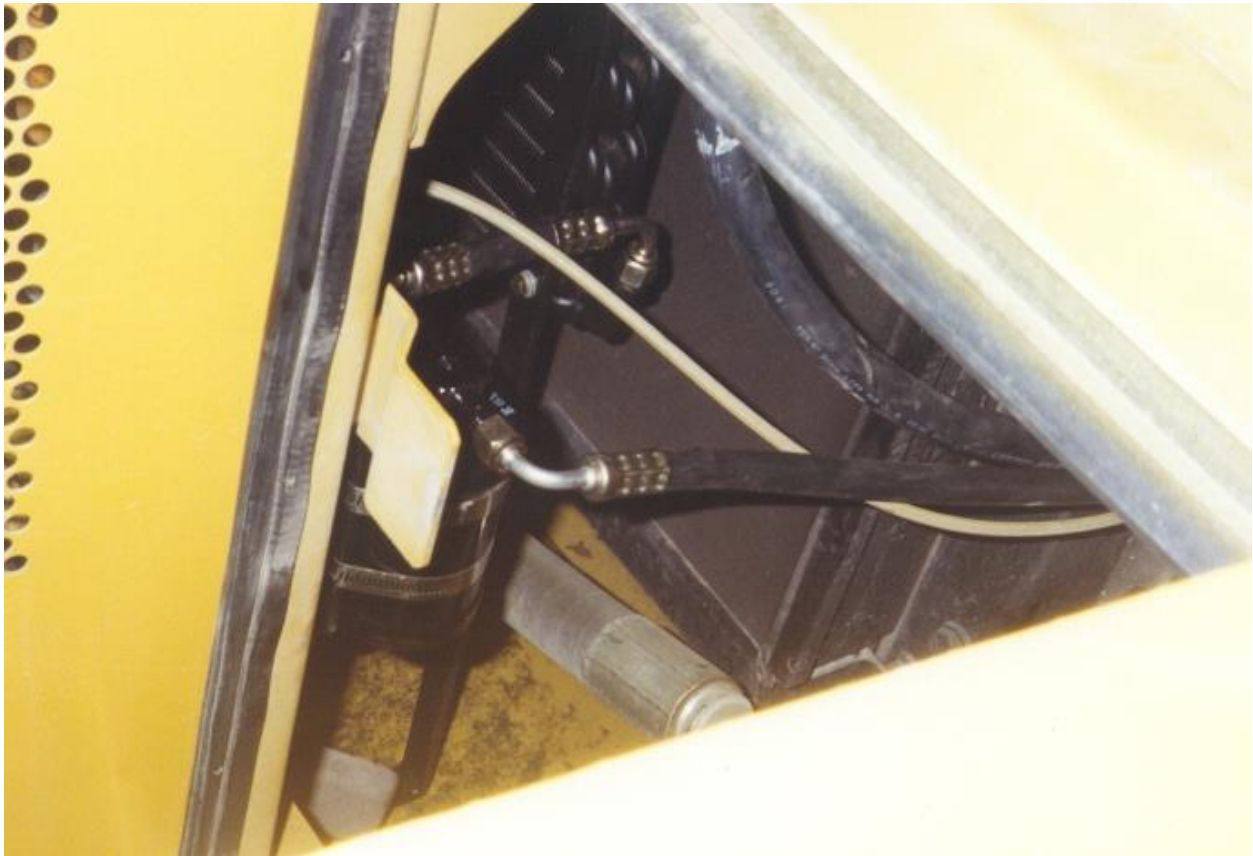
Drier in location with hose from condenser and other hoses in view.
